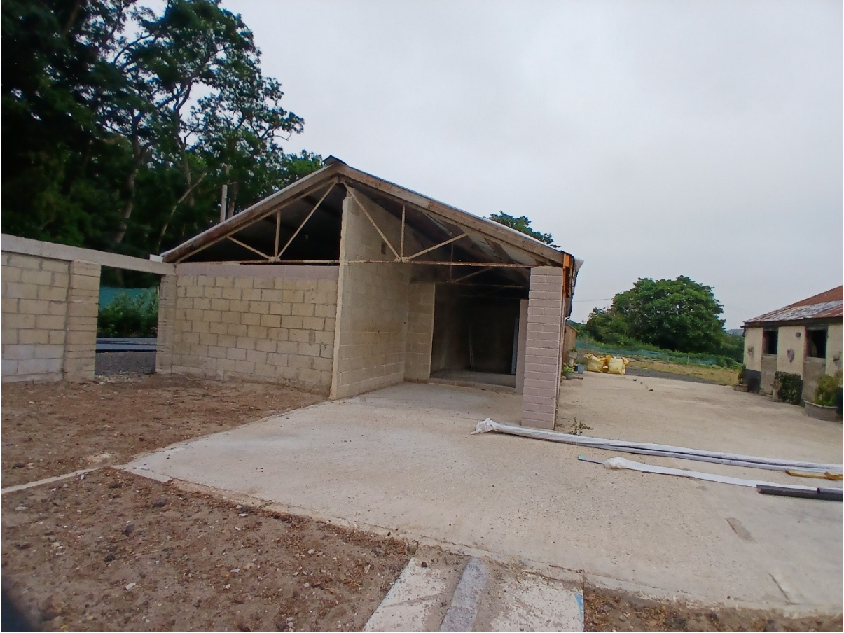
Figure 4: New southwest elevation showing the retention of the smaller southern stable block (right).
