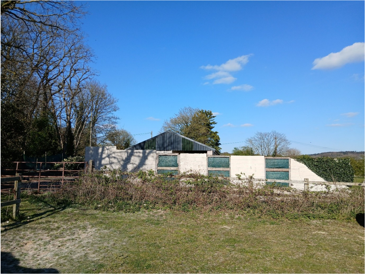
Figure 6: View of western elevation seen by "Solo Chase" taken by the Planning Officer. The original stable openings have been enclosed using fabric material with a timber frame. The appearance of this development no longer resembles equestrian use.
