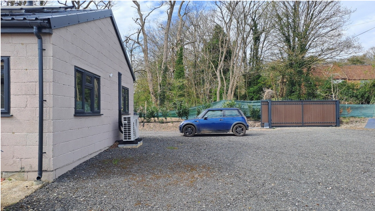
Figure 2: Residential component to the left (eastern elevation). New UPVC windows, new gutters and downpipe, air source heat pump. Tall impermeable entrance sliding gate to the north installed without permission.
