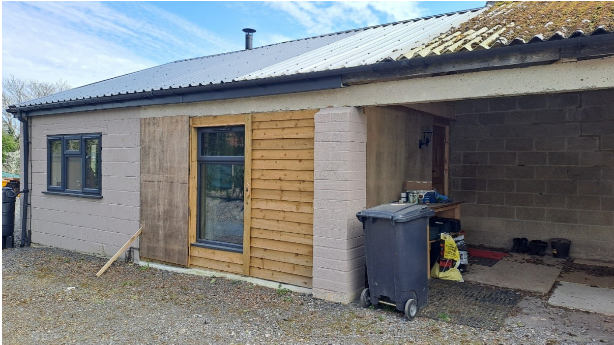
Figure 4: Rear elevation of residential component. New openings to the right for undercover parking, new roof sheeting, UPVC windows, guttering, paintwork, timber panelling and flue. Previous weathered roof above remaining stables.
