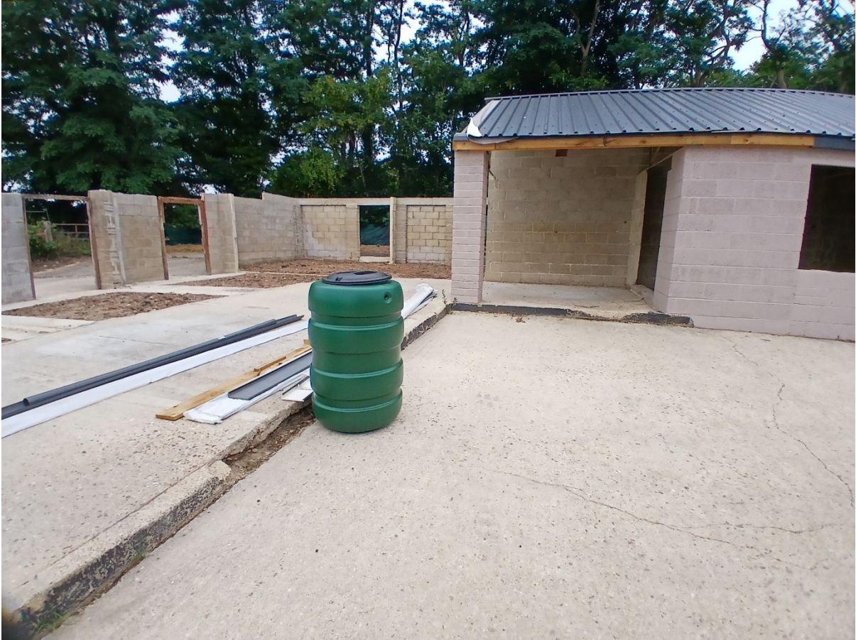
Figure 3: View of the demolished section of the L-shaped building. Stable openings still evident in the outer walls. Dwelling extension under construction.
