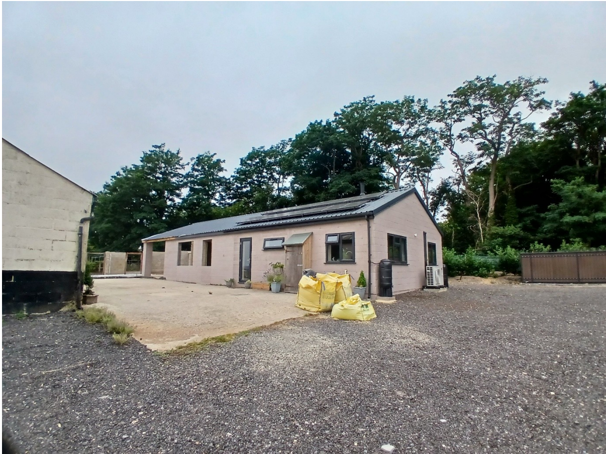
Figure 1: Southeast elevation of the former L-shaped building showing the residential component being extended into the remaining stall area shown on the plans. The walls have been painted and the roof replaced. Large areas of the L-shaped block have been demolished, with the outer walls retained for screening.
