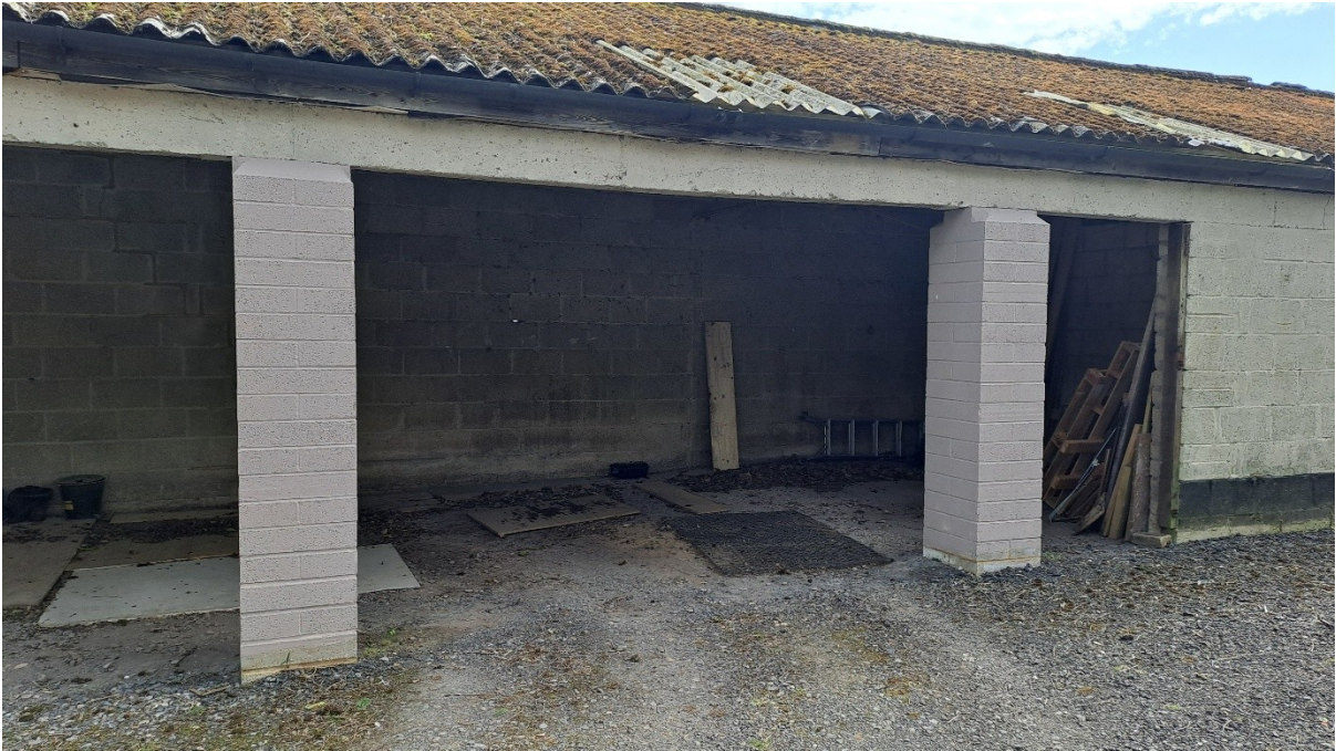
Figure 6: Rear side of stable area of northwestern building (southern elevation). Openings demolished and new structural pillars installed to open area for parking and storage. Weathered roof above. Unpainted stable areas to the right.
