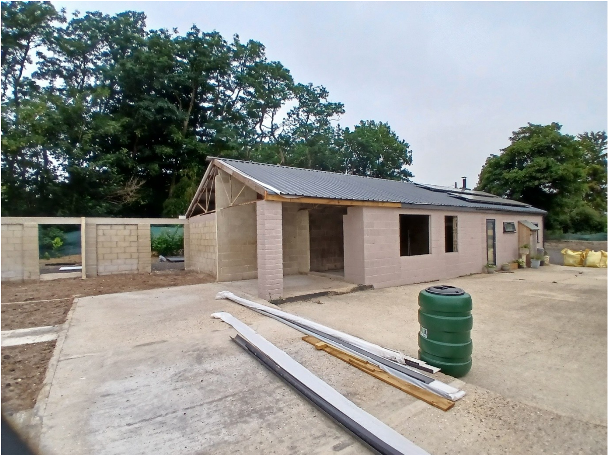
Figure 2: Southeast elevation where the demolition has taken place. An undercover seating area has been created with a new structural pillar installed. The stable openings have been closed with 2 new window openings installed. The dwelling appears larger than shown on the plans.
