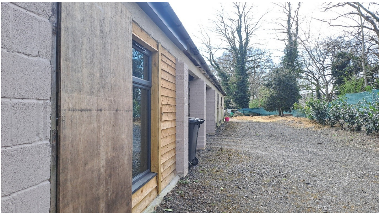
Figure 3: Residential component to the left (rear elevation) with the new openings for parking and storage. Stables are beyond. Sheeting material installed to the right along the by-way boundary.
