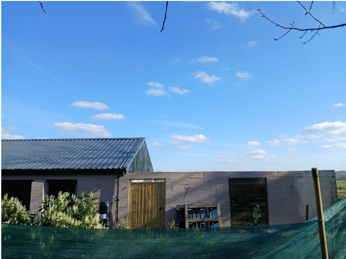
Figure 4: Northwest elevation of the demolished portion of the L-shaped building viewed from the By-Way looking south. Only the external walls adjacent to the boundaries remain. The previous stable openings have been enclosed using timber panelling.
