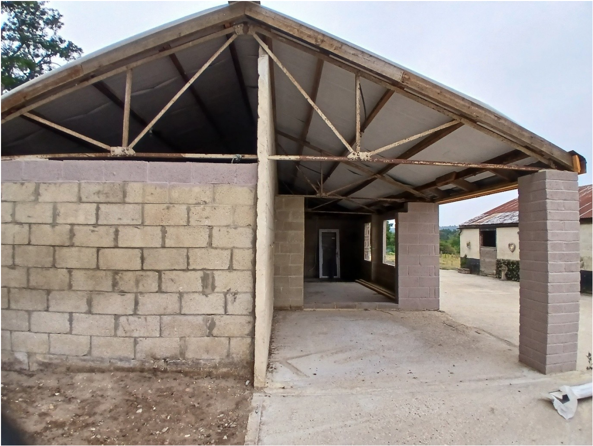
Figure 7: New southwestern elevation. Southern stable block to the right retained. New structural pillar and walls.
